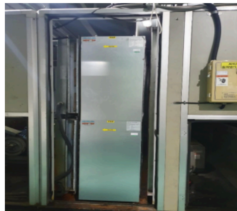
Heat-Pipe Pre Cooling System 설치 후
