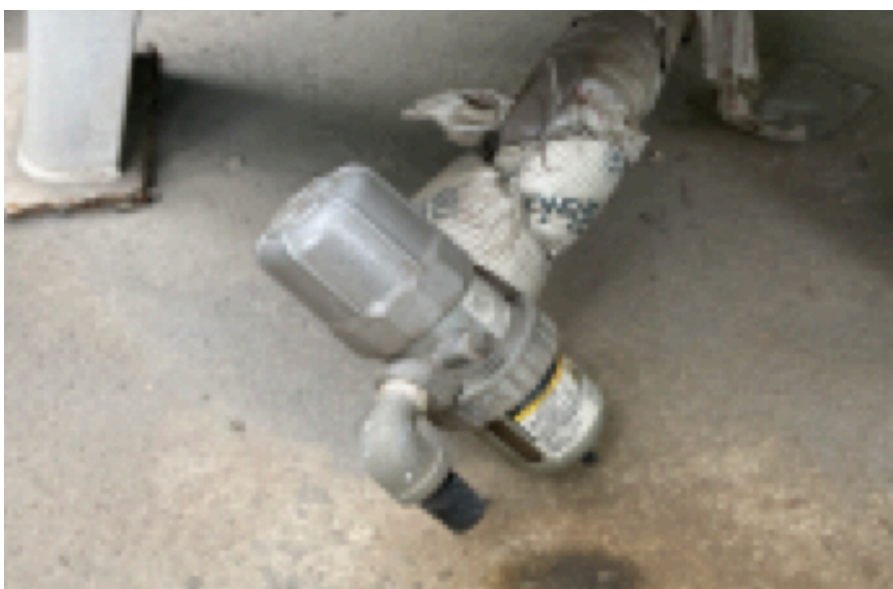
Receiver Tank Drain Trap
