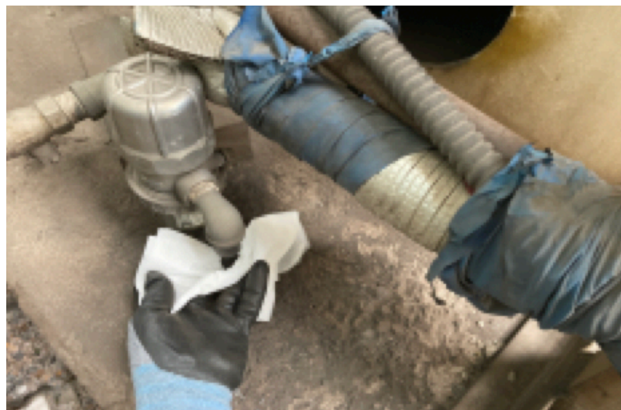
Receiver Tank Drain Trap
