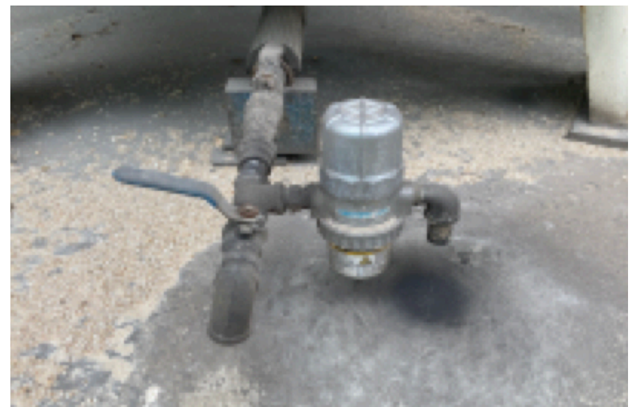
Receiver Tank Drain Trap
